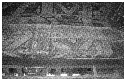
图7 2层3/④-⑥梁裂缝
